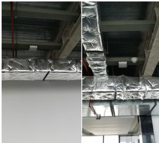
Figure 131: pRRUs of the test network installed on the ceiling.
