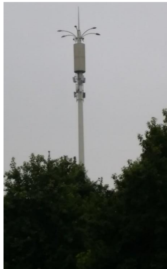
Figure 133: Outdoor 5G gNB outside the building.
